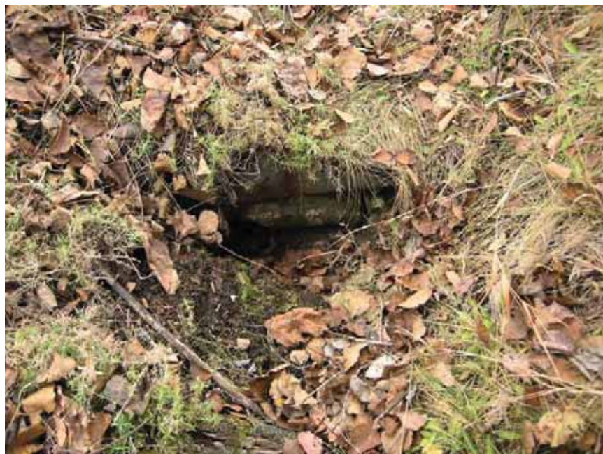
Figure 2.21. Grey water drain in kitchen/bath area.
